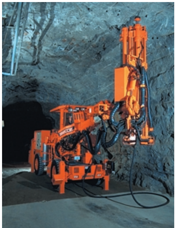
Underground: Tamrock Robolt drilling machine at work with Gardner Denver CT inside.
